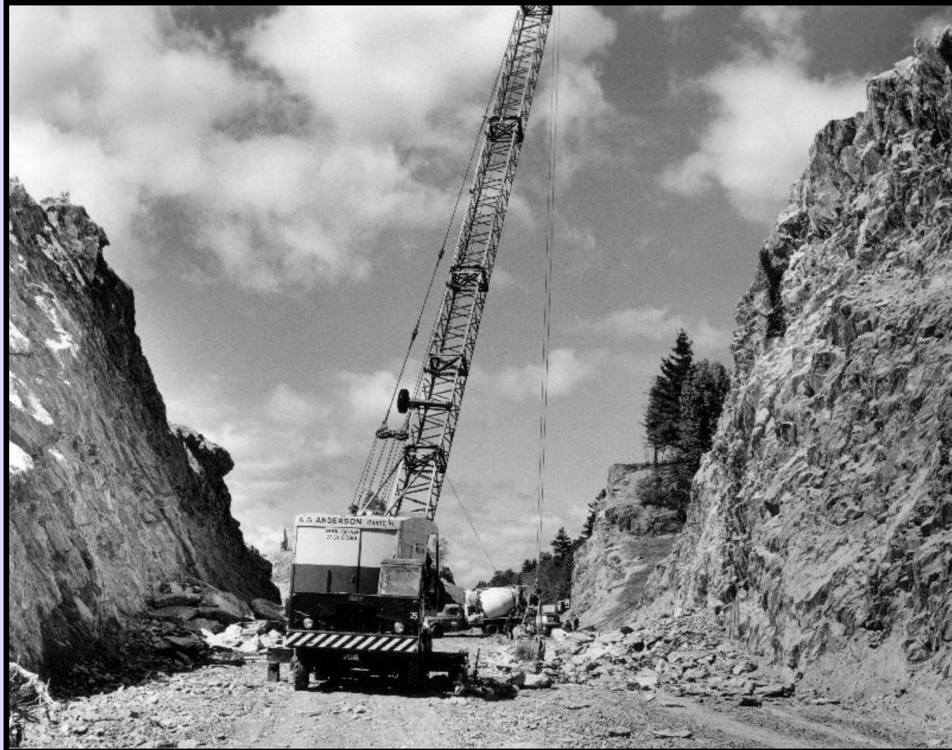
A crane and boulders rest in what will be Interstate 89 outside of Montpelier. 1959 (LS06102)
