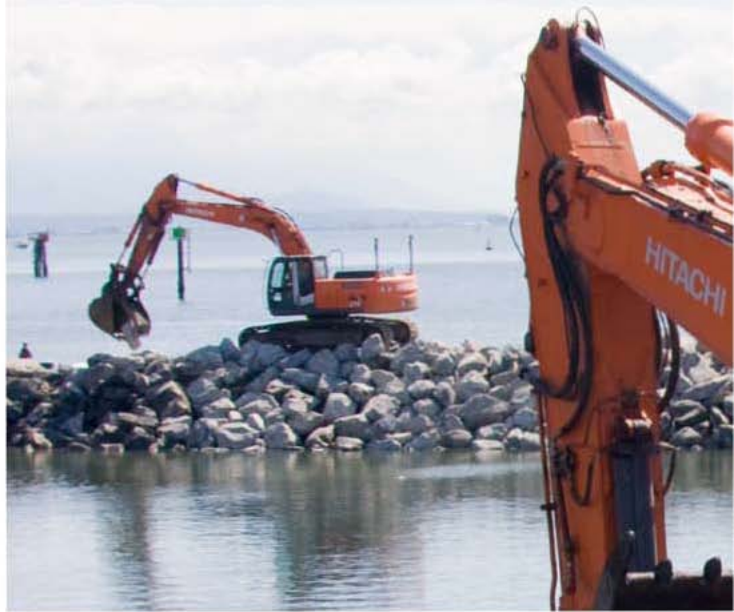
A Hitachi ZX270-3 is positioned on top of the breakwater to carefully key or lock the rock above the low tide line. The Hitachi ZX270-3 also has the same computer-based GPS screen and internet connectivity as the EX1200.
