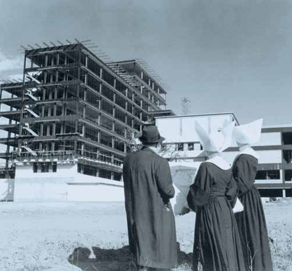
In 1962, two sisters of St. Paul's Daughters of Charity order, along with an unidentified man, observe progress on the steel frame of the new St. Paul Hospital under construction on Harry Hines Boulevard. The hospital opened in 1963.
