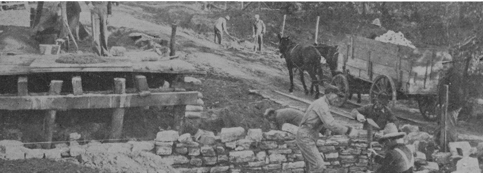
WPA workers constructing Teller Road in Johnson County, c.1935. Note the use of stone masonry.
