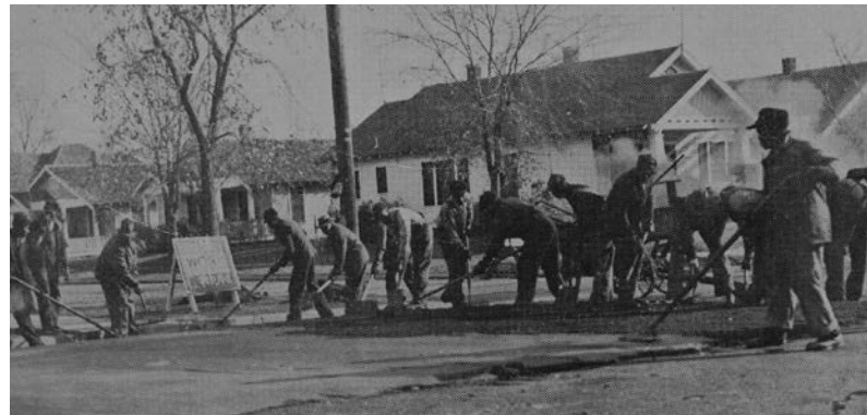
Workers repairing streets in Muskogee as part of a WPA project, c.1935.
