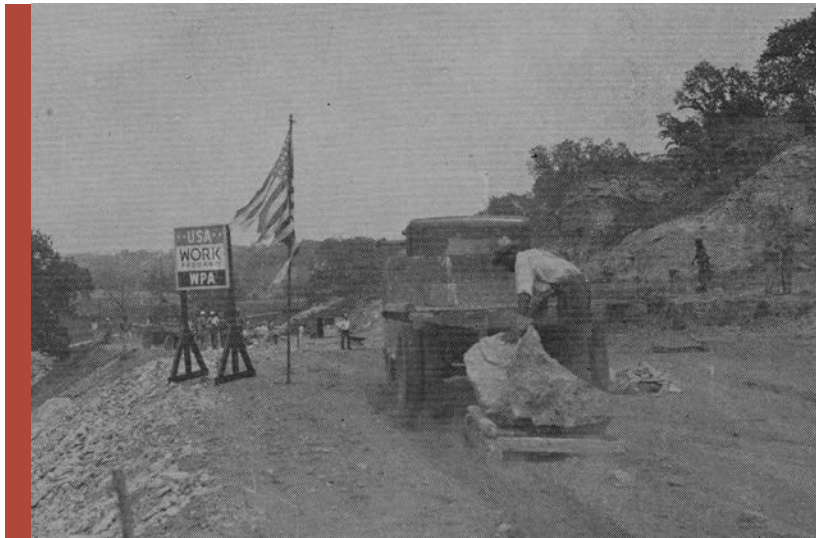
WPA workers construct a shortcut between Sand Springs and Tulsa, one of many projects that involved new road and bridge construction, c.1935.
