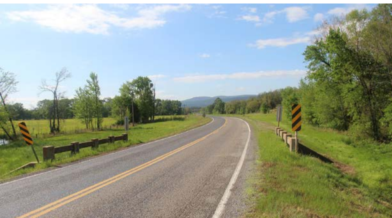
A typical WPA concrete culvert, as seen from the roadway, on State Highway 63 in Le Flore County (Structure No. 4040 1659 X).
