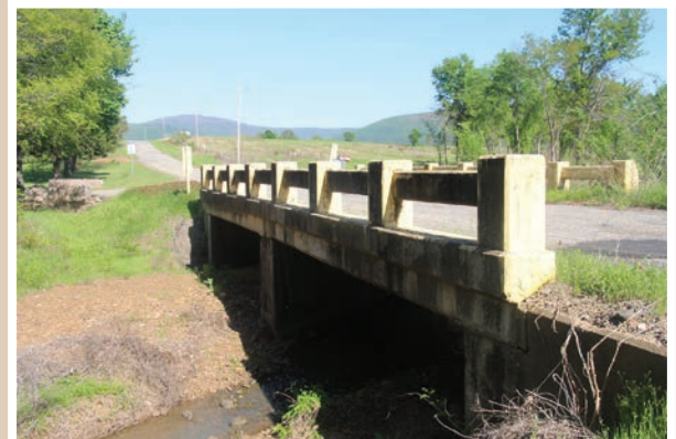
Both of these bridges are located in Le Flore County. The steel stringer bridge (Structure No. 4014 2619 X), constructed with U.S. WPGC funding, carries U.S. Highway 271 over an abandoned railroad, and the concrete slab crossing (Structure No. 40E1410N4810002) along County Road E1410 was built by the WPA.
