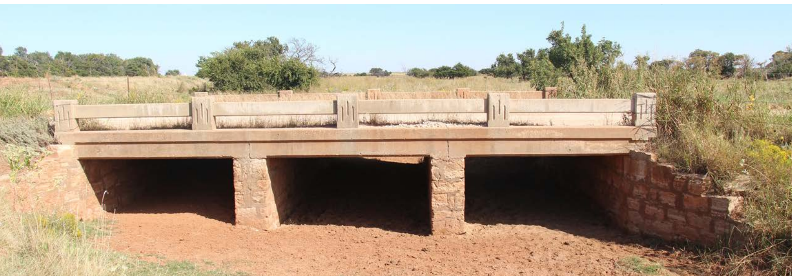
This 1938, WPA-built, concrete slab bridge in Blaine County was likely erected as part of a farm-to-market road project (Structure No. 06N2670Eo820002).
