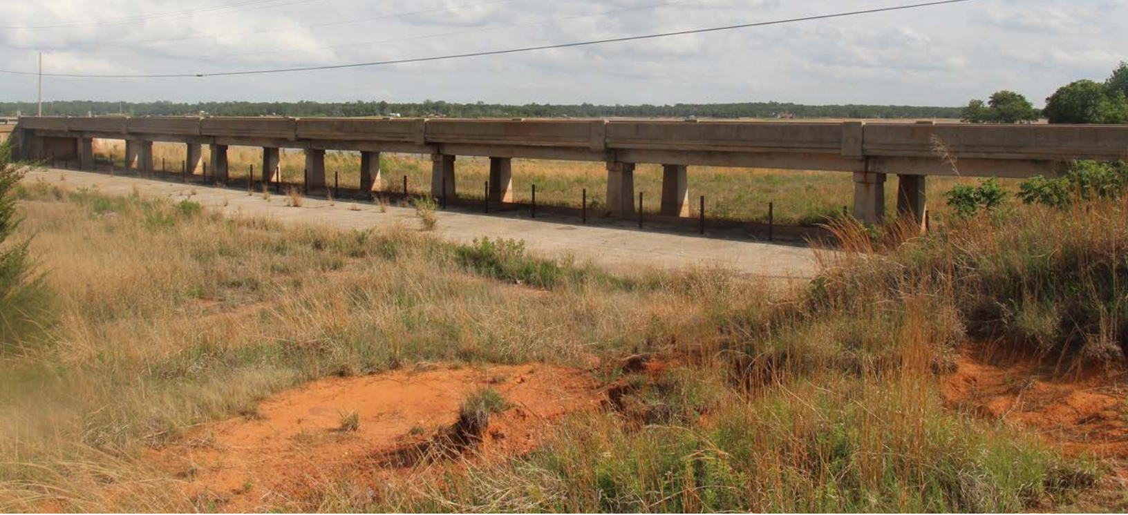
This concrete stringer bridge, built by the PWA, crosses the Shawnee Lake Spillway in Pottawatomie County (Structure No. 63E1150N3330002).
