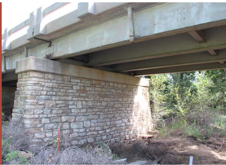
This steel girder bridge with a masonry substructure was built in 1940 by the WPA in collaboration with the local Beaver County government (Structure No. 04E0140N1320008).
