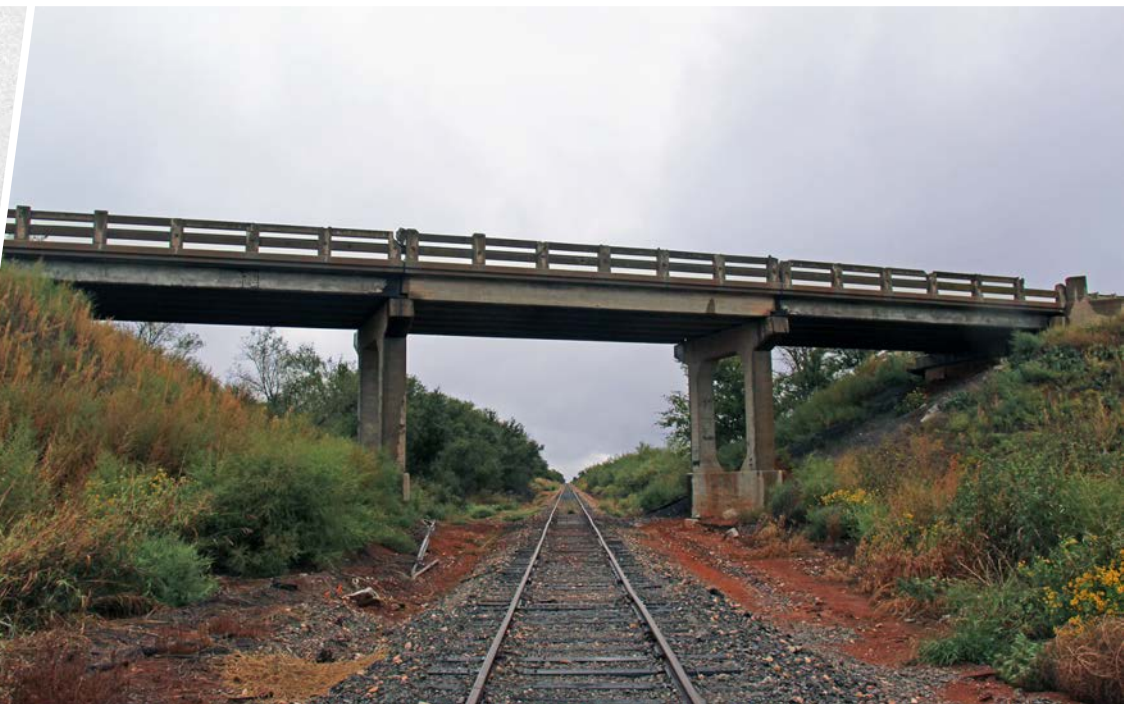
The WPGC funded this steel beam and girder bridge in 1936 to carry State Highway 152 over the railroad line in Washita County (Structure No. 7508 1345 X).
