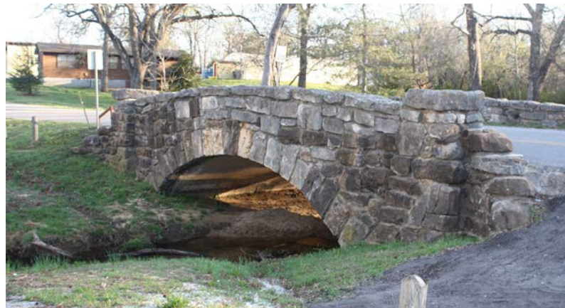
This stone arch bridge in Wintersmith Park, constructed in 1934 by the CCC, represents the agency's extensive road and bridge building within parks (Structure No. 62N3570E1550001).
