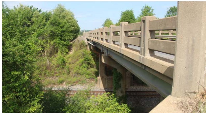
A railroad overpass in Le Flore County, originally constructed with WPGC funding, which demonstrates the lasting importance of Depression-era roads and bridges throughout the state (Structure No. 4042 0015 X).
