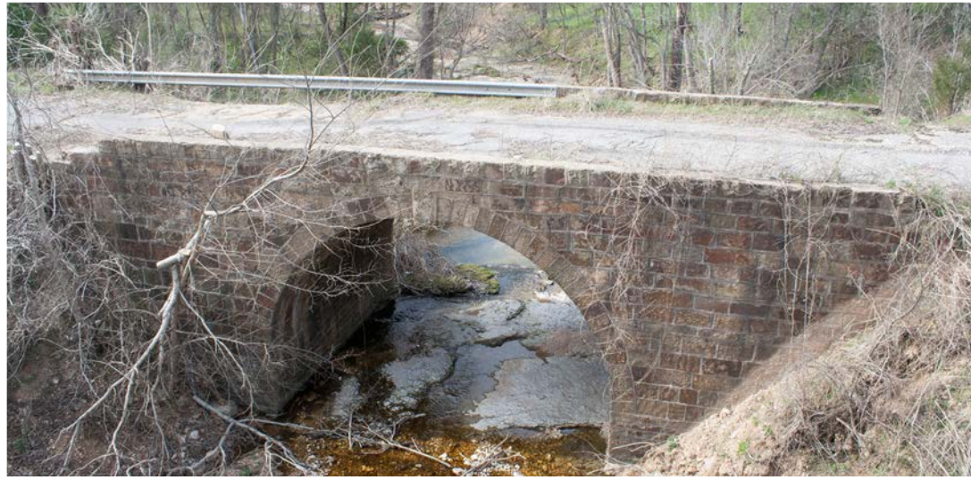
This limestone arch bridge was constructed in Mayes County in 1930 by members of the nearby Cherokee tribe using federal funding through the Bureau of Indian Affairs. Projects like this were precursors to the CCC-ID (Structure No. 49E0610N4390007).
