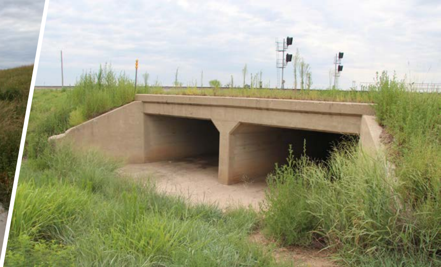
This culvert along State Highway 15 was built using NRWR funding (Structure No. 2320 0451 X).
