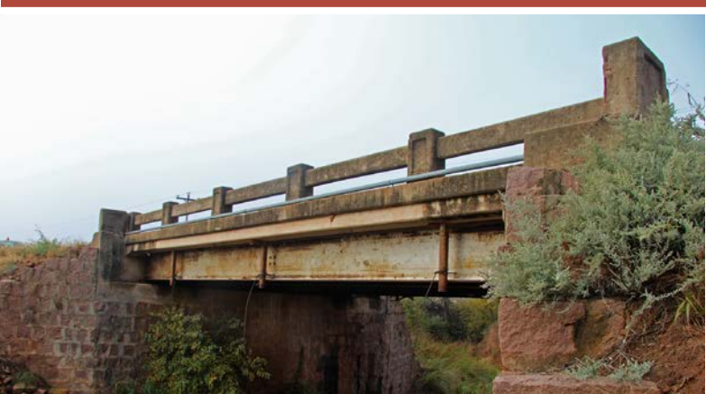
This 1941 steel girder span, characteristic of many steel bridges constructed for small crossings, was built by the WPA in Greer County (Structure No. 28N1840E1390009).
