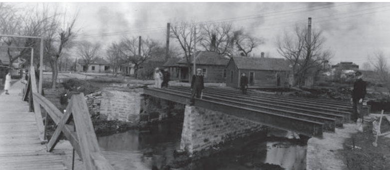
CWA employees in Okmulgee reconstructing a bridge, which was a common form of relief work, 1933.
