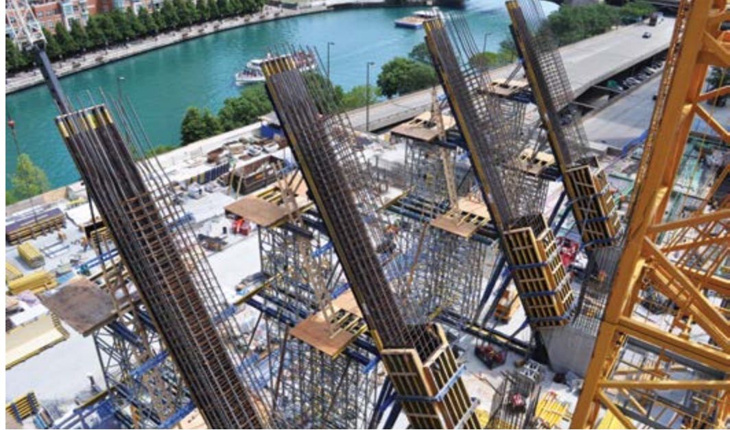
Figure 7. Angled columns support the thrust of the hotel portion of the project and carry it over the street, making for a distinctive volume with large interior spaces.
