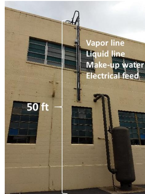
Vapor and Liquid lines
