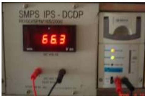
Fig.:6 Measurement of output voltage of DC-DC converter
