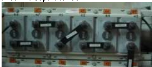
Fig.:9 VRLA battery bank
