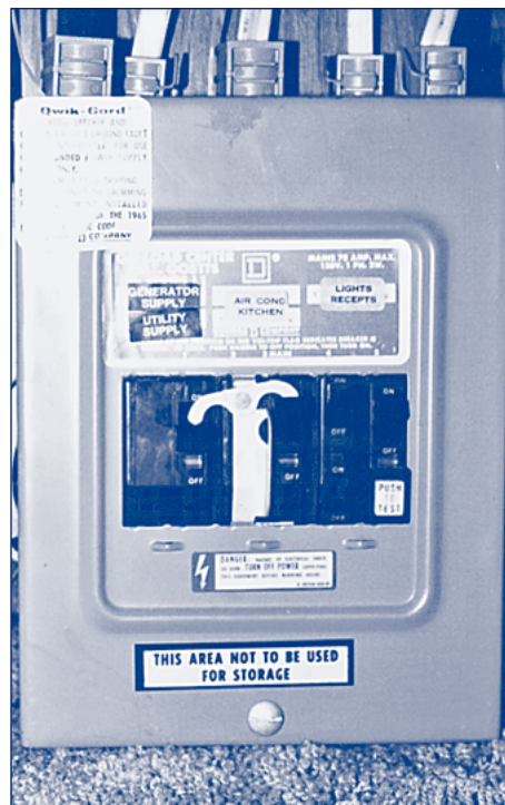
A Royale 30-amp, 120-volt AC panel with two main breakers and a flipper. The breaker with the flipper can be eliminated with an automatic transfer switch.
