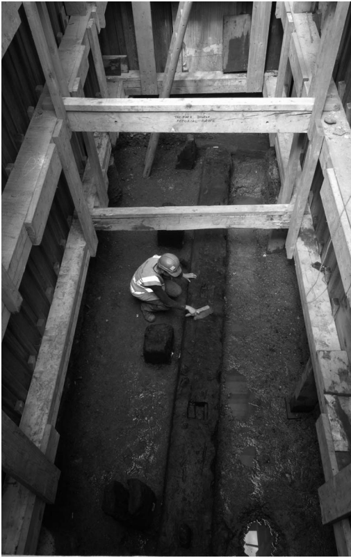
Fig 3. The basal tier of the baulks of the second phase of the Late Roman quay, view looking west. There are driven piles to the south of the quay baulk (Maggie Cox, MOLA)
