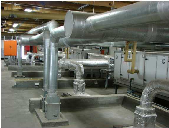
Air ducting and air handling units
