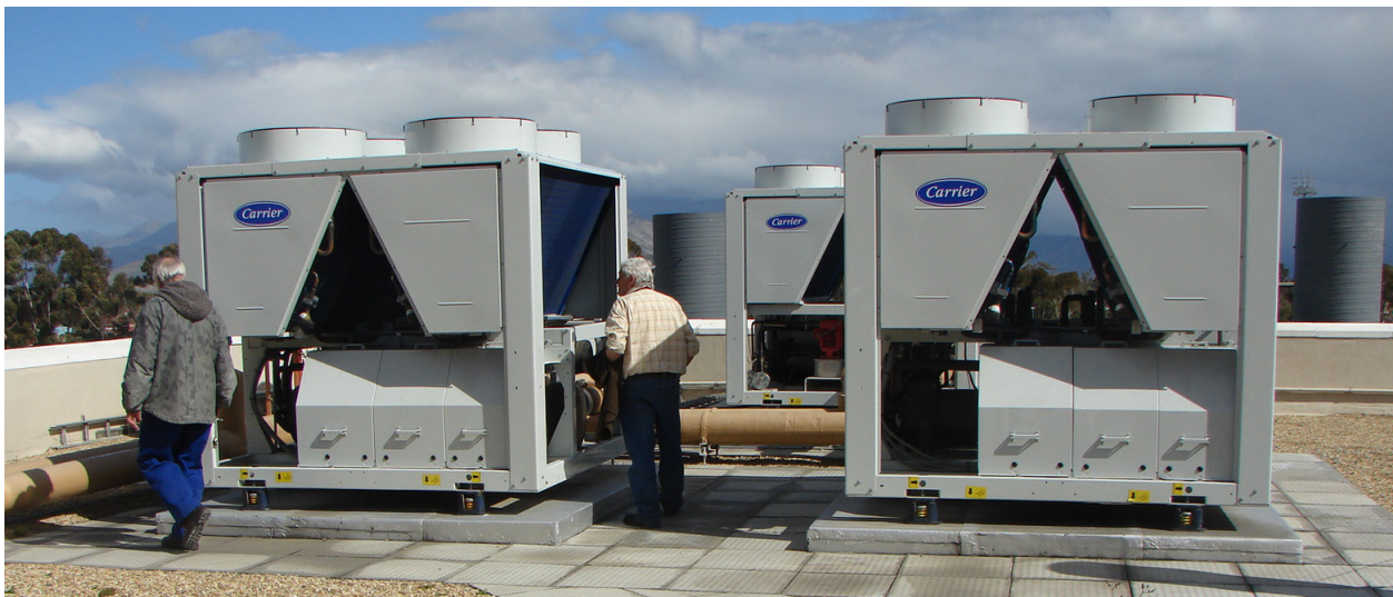
Air cooled chiller – heat pumps
