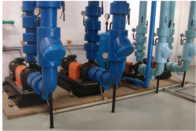
Chilled water pumps
