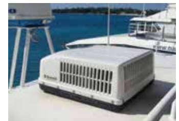
Dometic's DuraSea Rooftop installed on a Bahamas Ferries Sealink catamaran.
