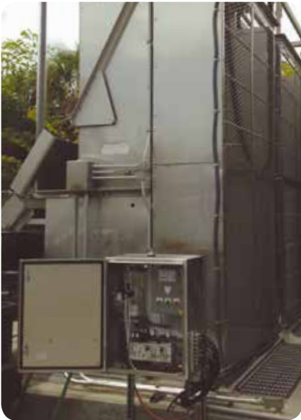
Waste water treatment
