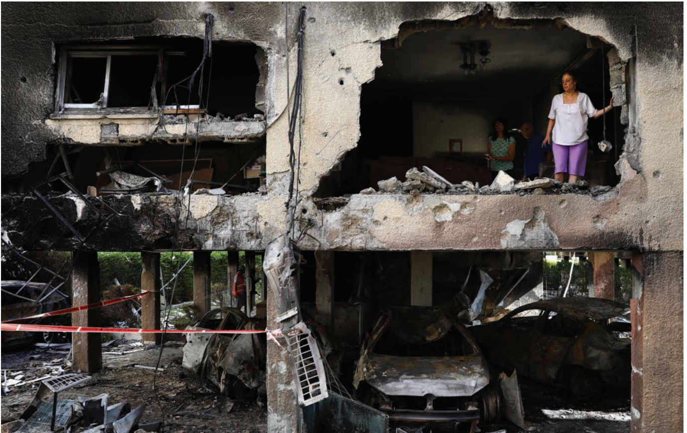
Members of the Srour family inspect the damage of their apartment in Petah Tikva, Israel, after it was hit by a rocket fired from the Gaza Strip on May 13.
