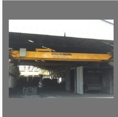
Double Girder Overhead Crane
