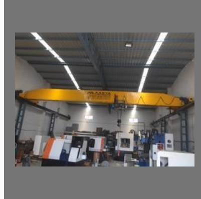
EOT Overhead Crane
