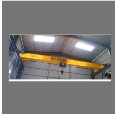
Overhead Traveling Crane
