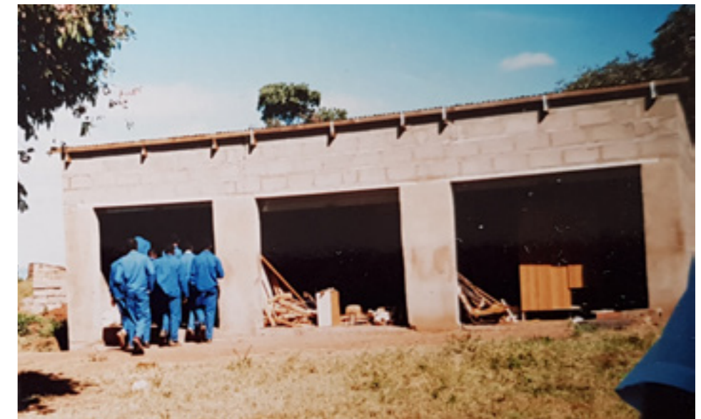
Training young Mafucula residents in construction. The building of the micro-enterprise centre involved training young Mafucula residents in construction skills
