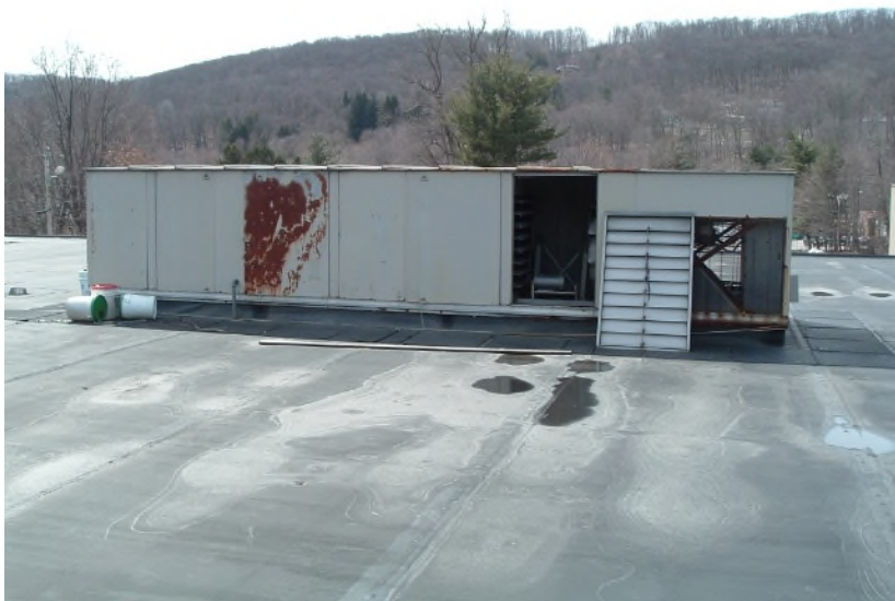
Existing Lennox unit
