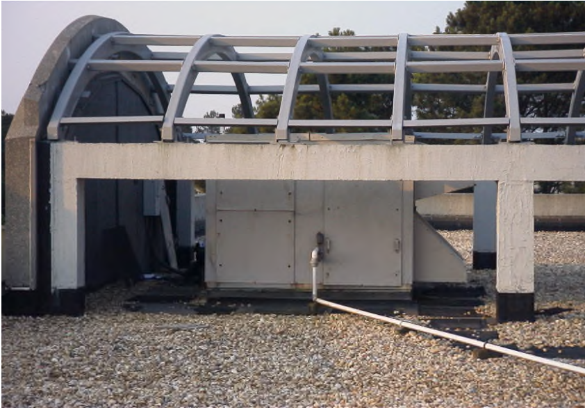
Existing York unit
