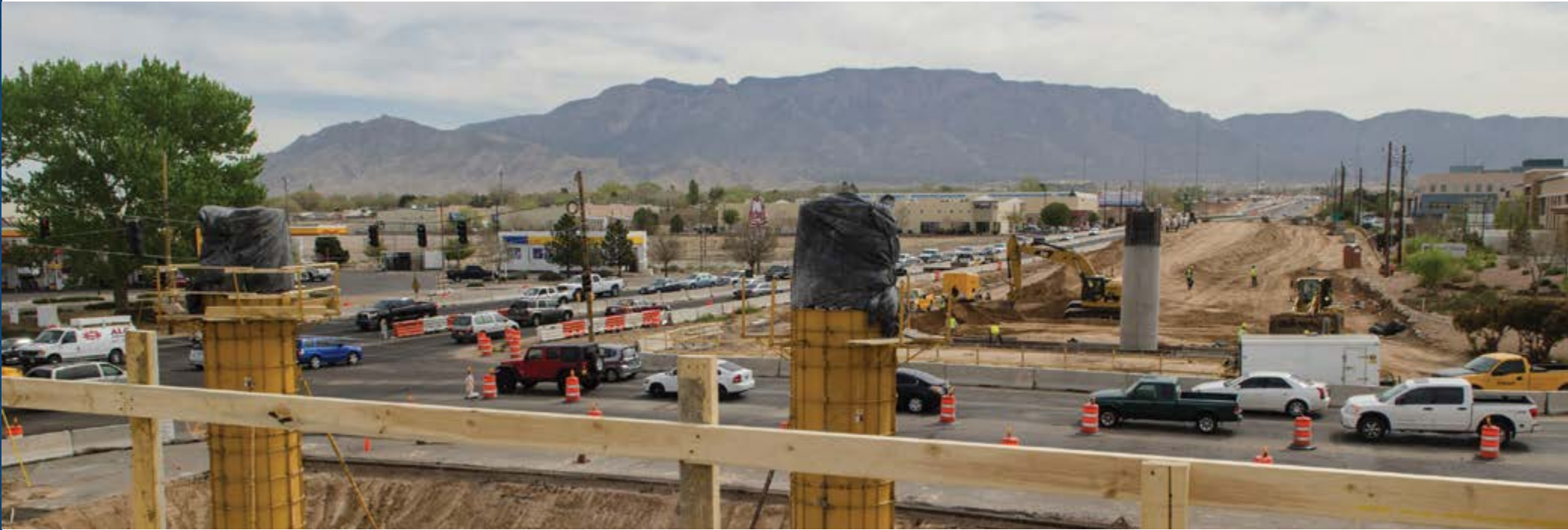
Construction on the Paseo del Norte/I-25 Interchange Reconstruction Project (Photo courtesy of Wilson & Company)
