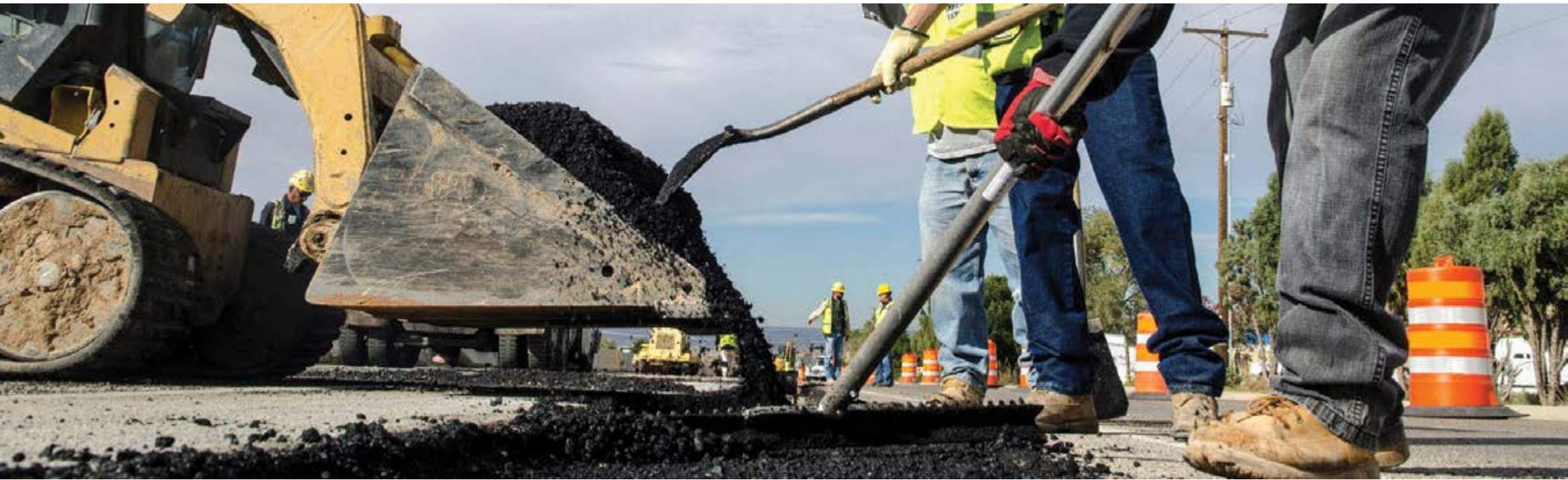
Construction on the Paseo del Norte/I-25 Interchange Reconstruction Project (Photo courtesy of Wilson & Company)
