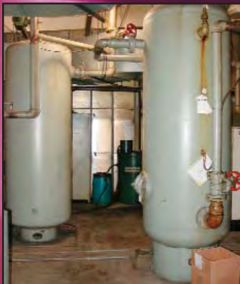
VIEW OF RECEIVER TANKS
