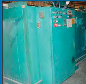
OSI CURING OVEN, GAS FIRED
