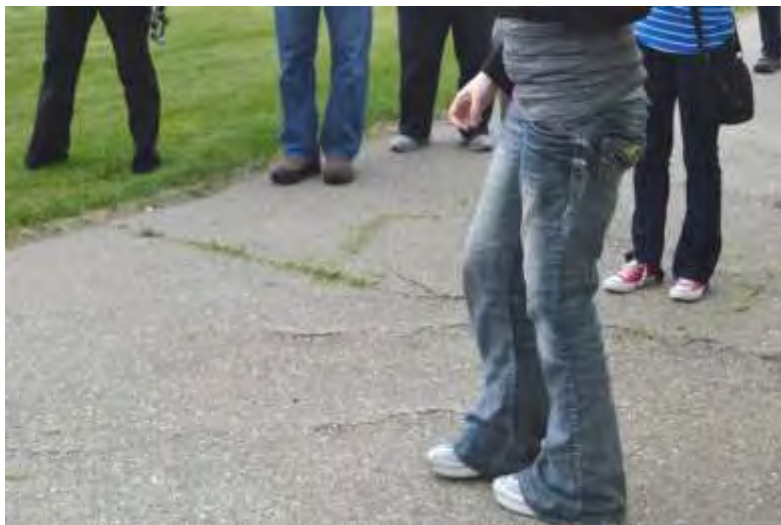
Figure 6: Tree roots pushing up asphalt trail west of wetlands overlook. Photo courtesy Marylu Dykstra, Disability Advocates of Kent County.
