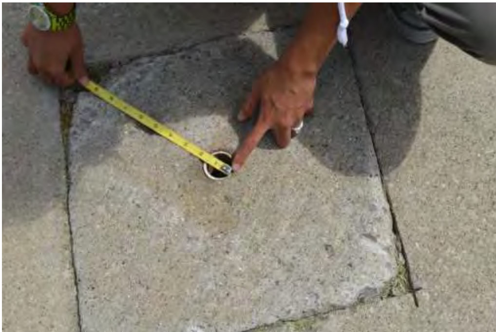
Figure 10: Hole in sidewalk after removal of stanchion. Photo courtesy Marylu Dykstra, Disability Advocates of Kent County.
