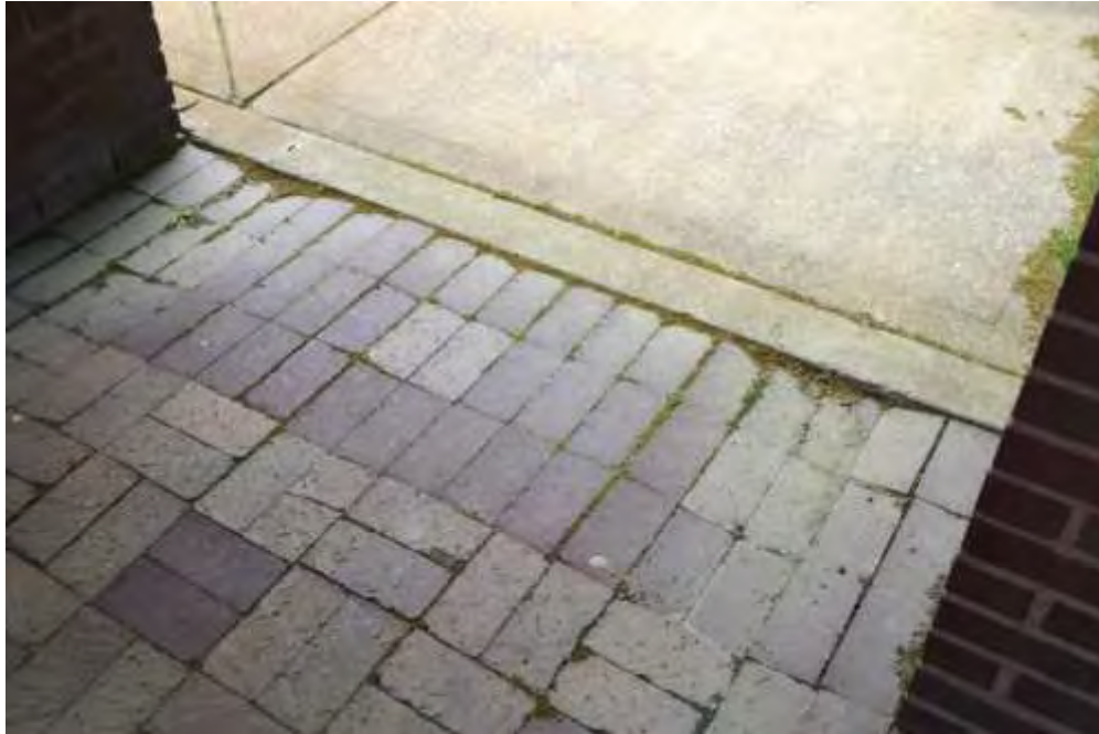
Figure 9: Brick sidewalk requiring repairs. Photo courtesy Marylu Dykstra, Disability Advocates of Kent County.
