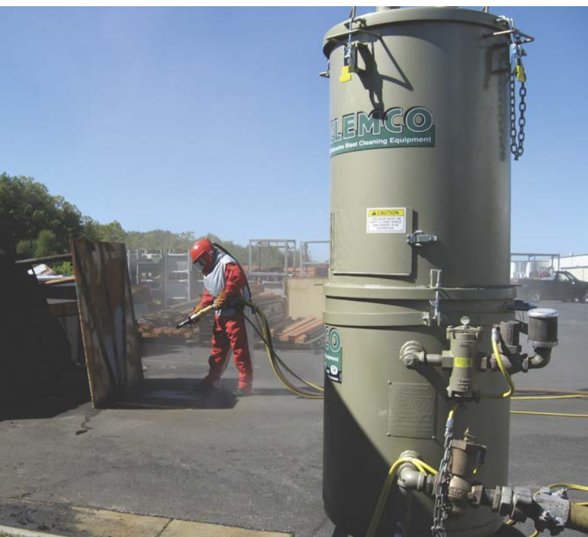
Fig. 1: Effective and safe abrasive blasting requires the correct equipment and setup as well as a properly trained operator. All figures and tables are courtesy of Clemco Industries.
