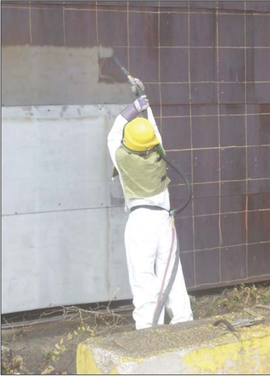
Productivity test, conducted under third-party guidance, on heavily pitted and rusted steel structure at a steel mill. Round and angular abrasives were tested for productivity and usage.
