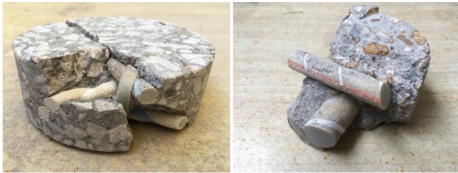
Fig. 5—GFRP coupons extracted from the concrete cores of Walker (left) and Southview (left) Bridge
