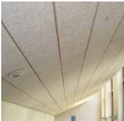
▲ Grace Church (New York, NY) Direct-Attached Ceiling Panels
