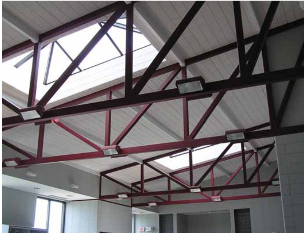
▲ Carlisle County High School (Bardwell, KY) Tectum V-Line Ceiling Panels
