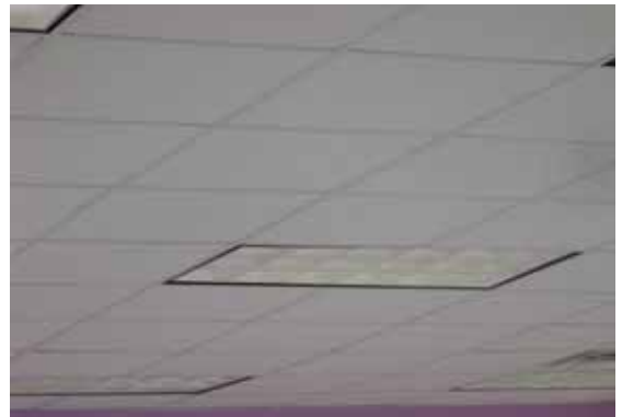
▲ Morningside Children's Academy (Oak Park, IL) Variations Lay-In Ceiling Panels
