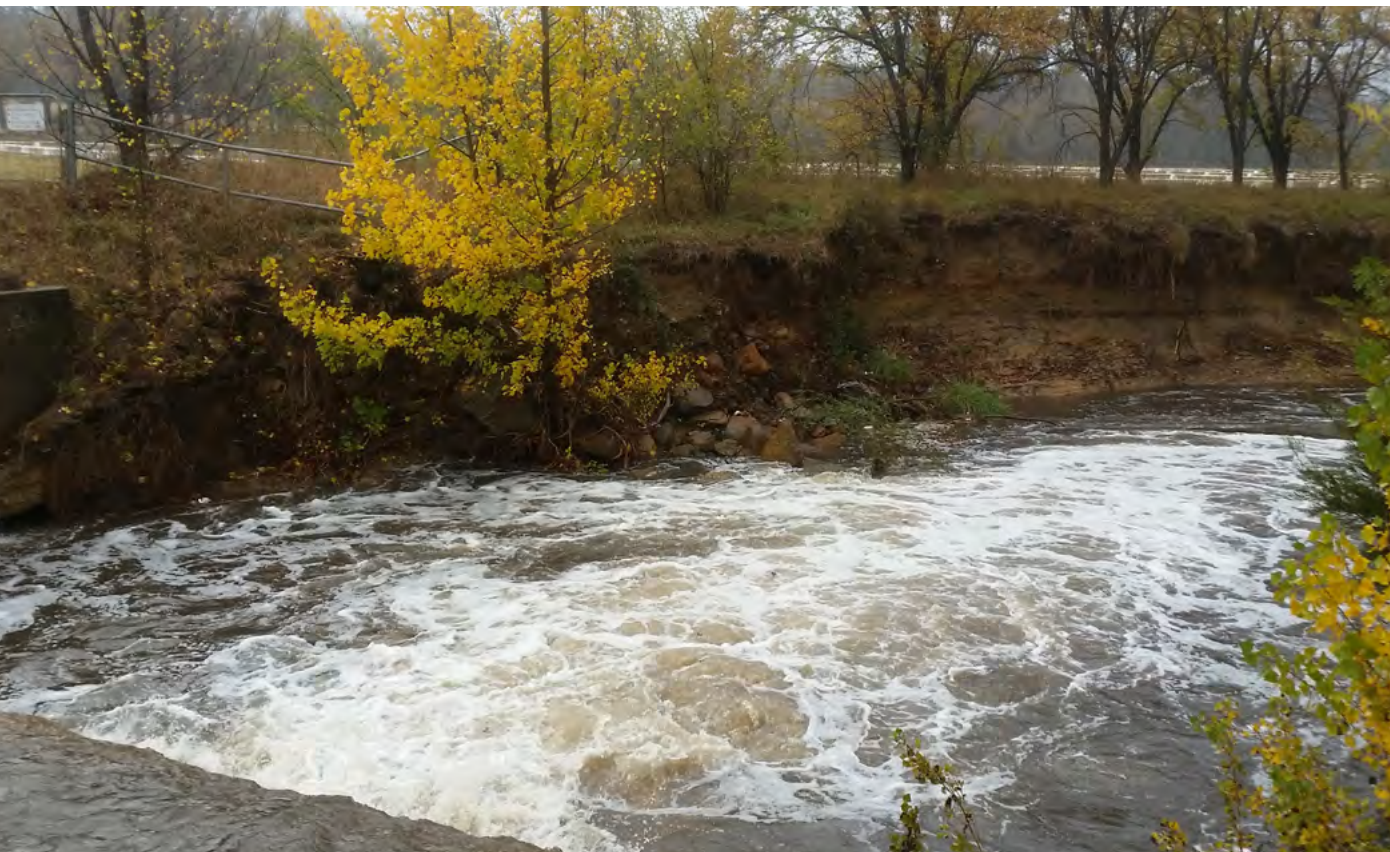
Erosion downstream of the Cotter Road on Yarralumla Creek during heavy rain
