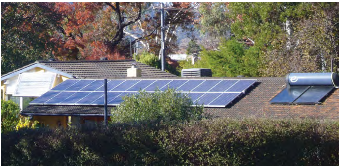
Residential roof top solar hot water and solar panels in Canberra
