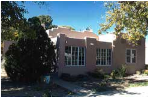
Zephyr Butler reroofed an historic home in Las Cruces, casting them from a mold he made from an intact tile.
