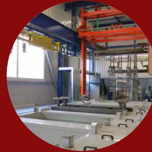
Pre Treatment 9 Tanks with PLC based Transporter
