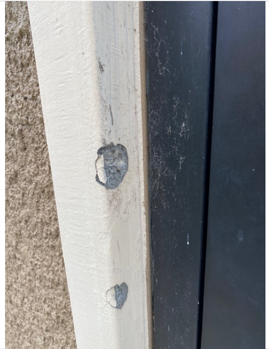
Damaged concrete trim
