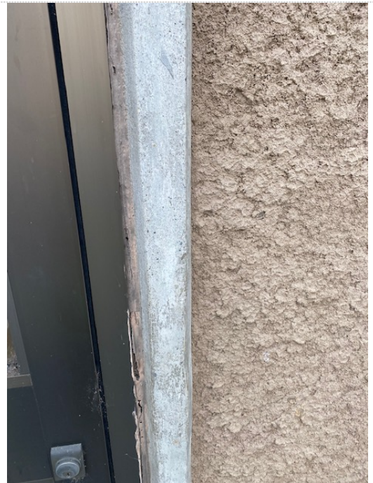
Damaged asbestos brown frame sealant-Building 1800A
