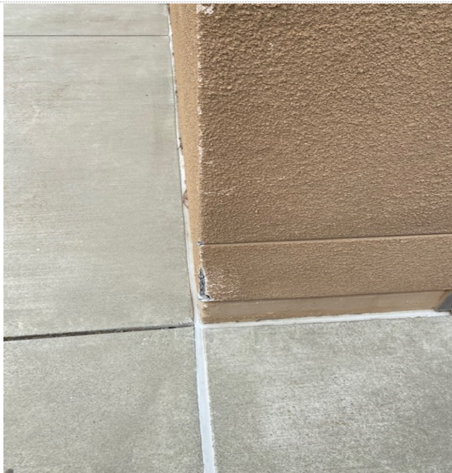
Damaged stucco at corner of Building 1400-Staff
