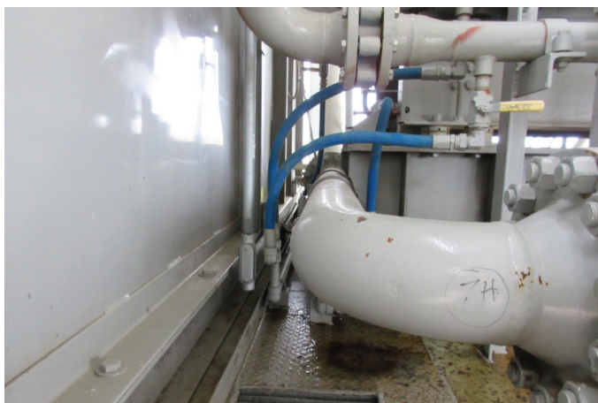
Figure 16. Left-Side Discharge Pipe Elbow
