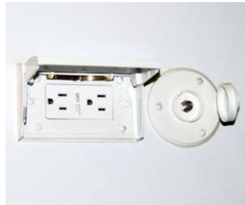
Indoor/outdoor satellite and cable connection
