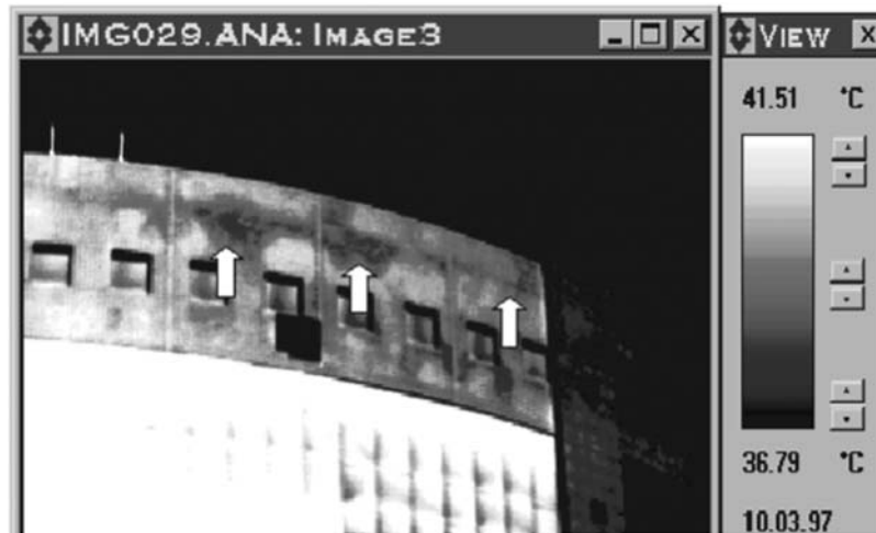
Figure 8-49 The lower-temperature areas (indexed by upward arrows) indicating the defected areas filled with water or moisture
