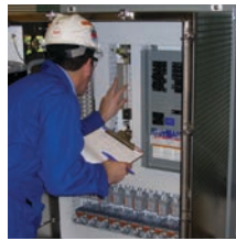
Control and Monitoring
