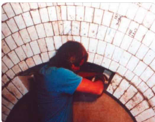
Sulphur recovery unit - head
