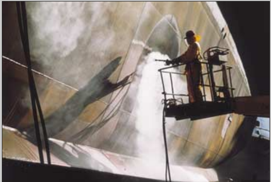
Shipyards make up the largest group of users of UHP waterjetting for surface preparation. Courtesy of Flow International and Todd Shipyards
