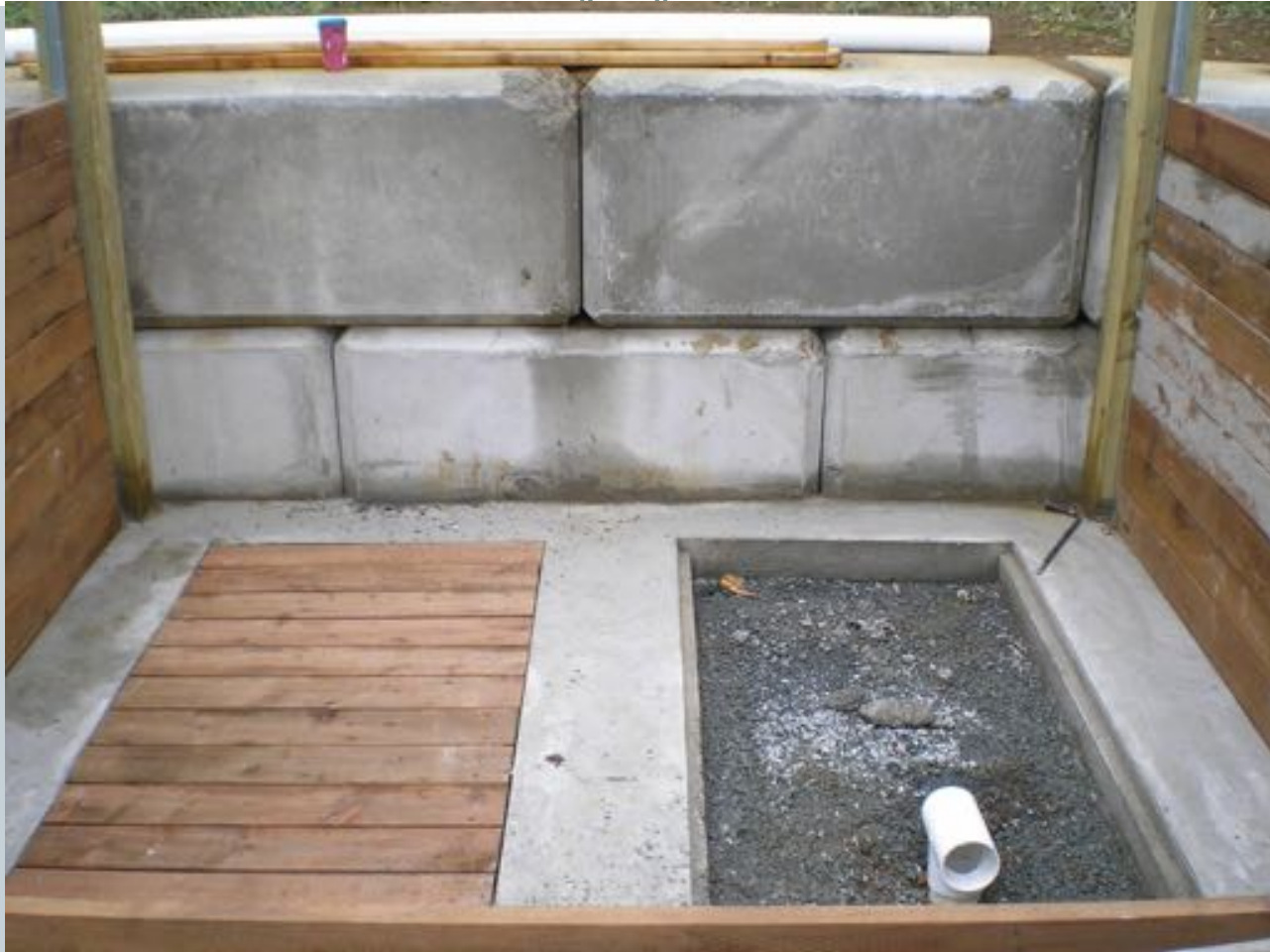
Completed Aeration System
