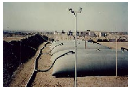
Figure 15. Generator Fuel Storage Bladder.
