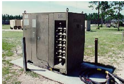
Figure 19. Secondary Distribution Center.
