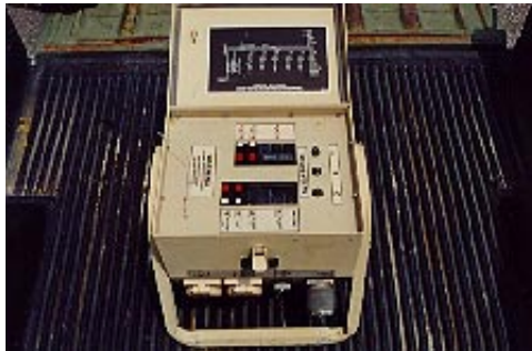
Figure 16. Facility Distribution Panel.
