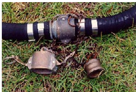
Figure 8. Water Distribution Hose.
