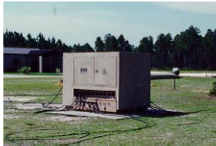
Figure 18. Primary Distribution Center.
