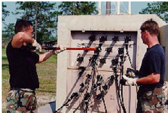
Figure 20. Primary Electrical Cable.
