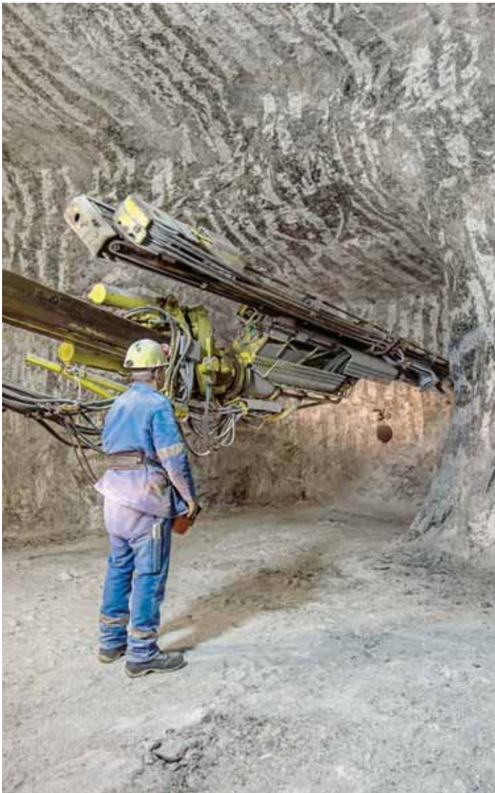
PREPARATION: A miner operates a 7-metre drill that makes holes for blasting in the Stetten Salt Mine in Germany. The drill is mounted on its own vehicle.
