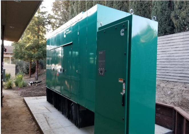
F. Civic Center Emergency Generator
