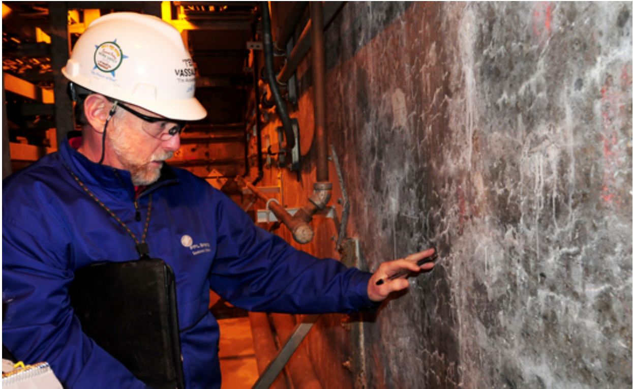
Figure 7 - Alkali Silica Reaction of Concrete at Seabrook Station
