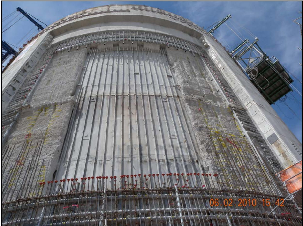
Figure 6 Crystal River 3 attempt to repair damage
