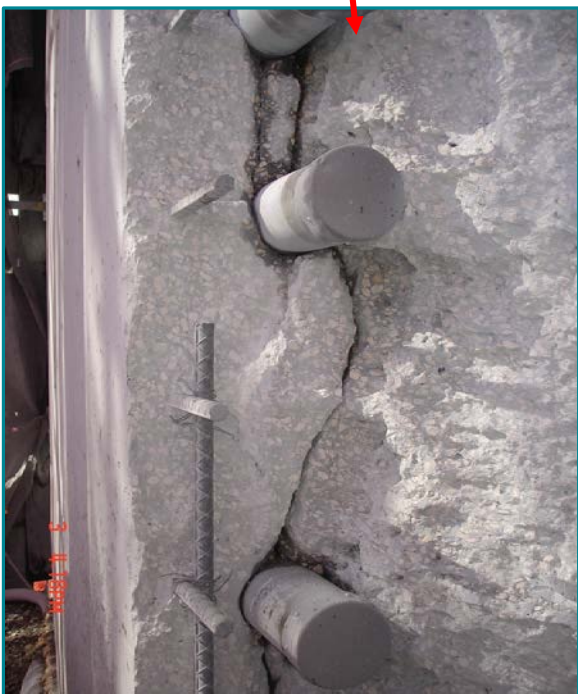
Figure 5 Delamination damage in Crystal River 3
