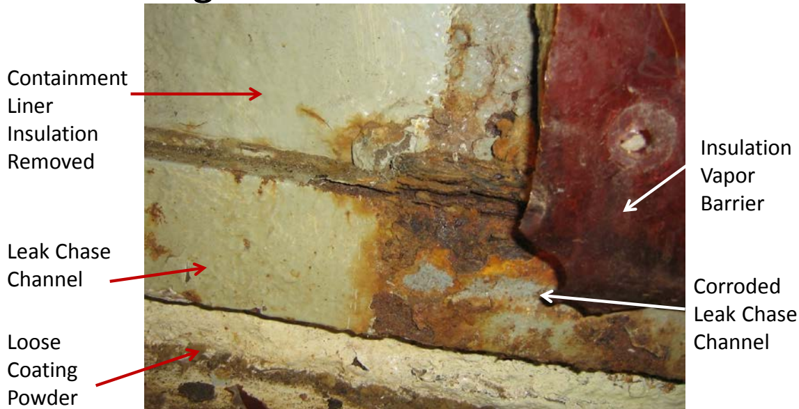
Figure 9 – Containment Liner Plate Corrosion
