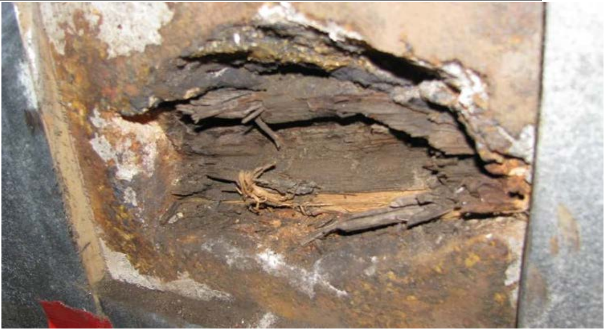
Figure 10 –Beaver Valley - Piece of Wood behind the Liner Plate
