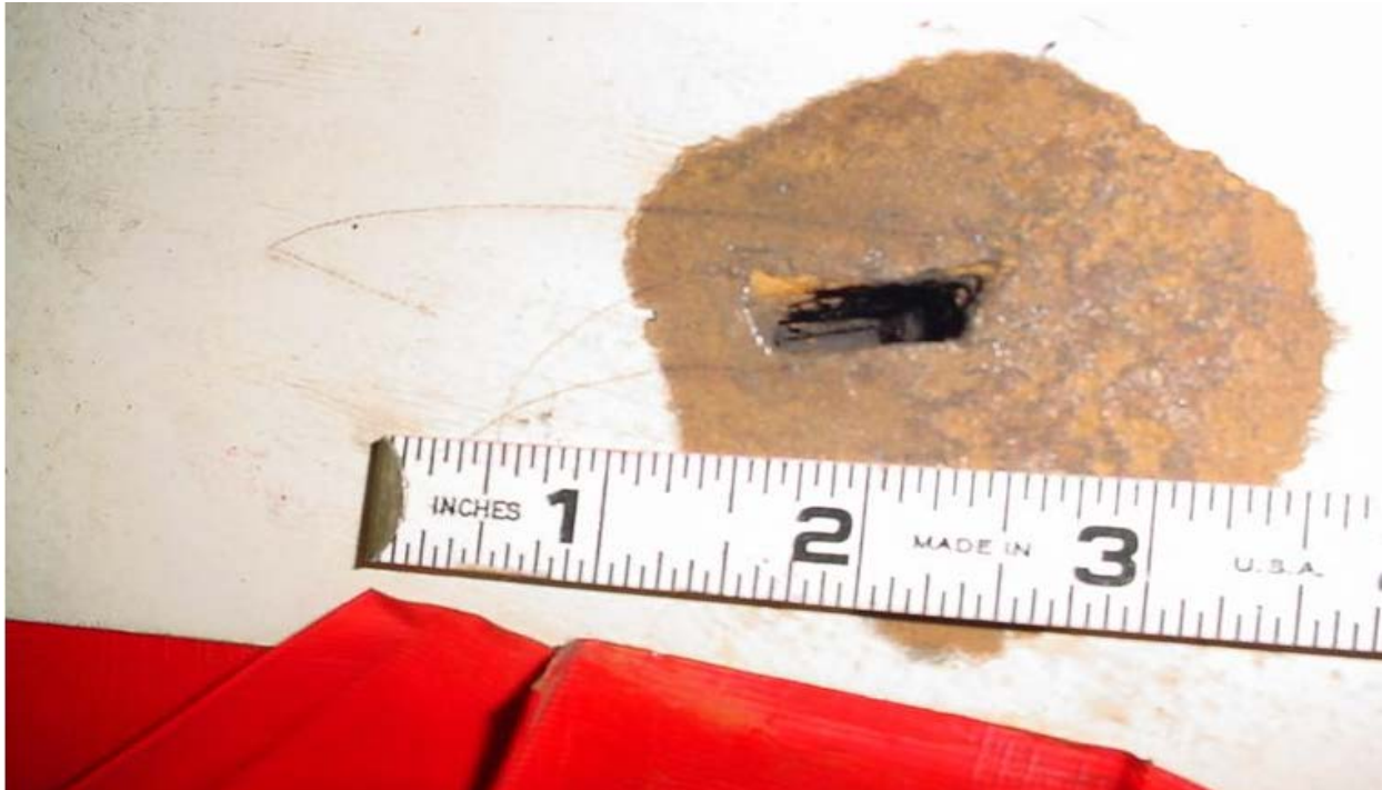
Figure 11 – Perforation of Liner at Beaver Valley
