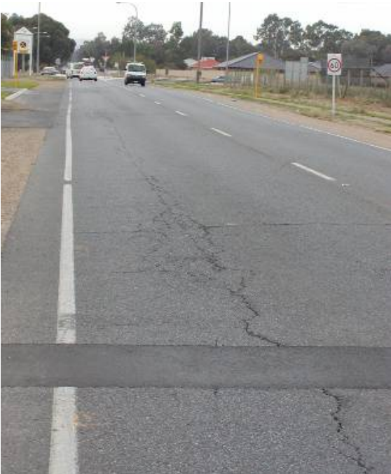
Figure 7.14: Longitudinal shrinkage cracks
