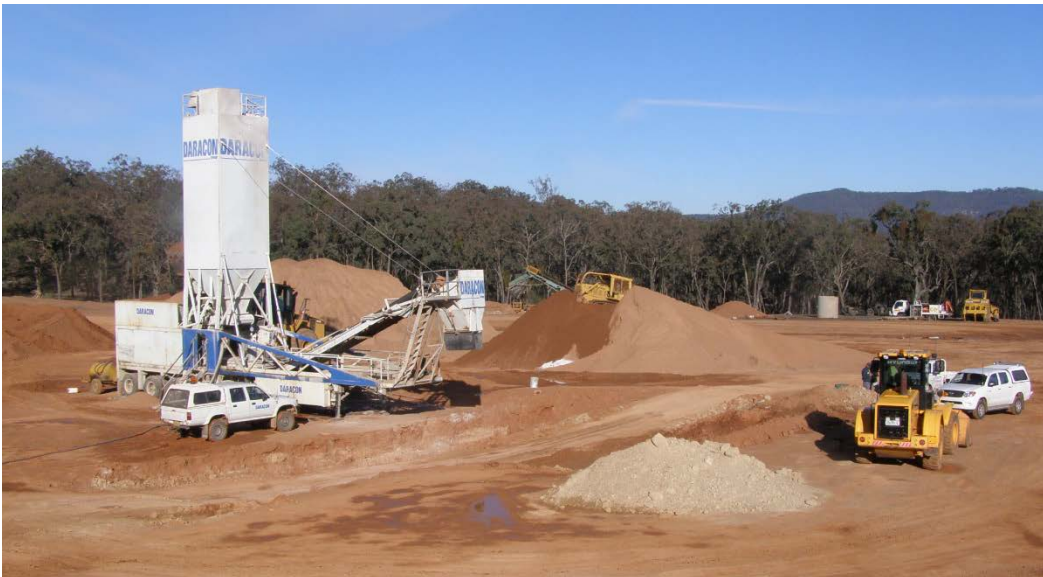
Figure 6.1: Typical pugmill used in a quarry for processing granular materials
