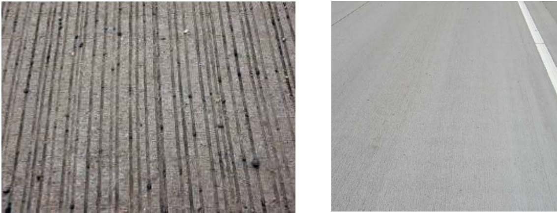
Figure 10.15: Tyned concrete surface
