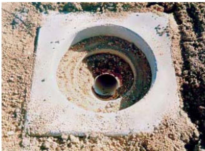
Figure 5.8: Pit with debris
