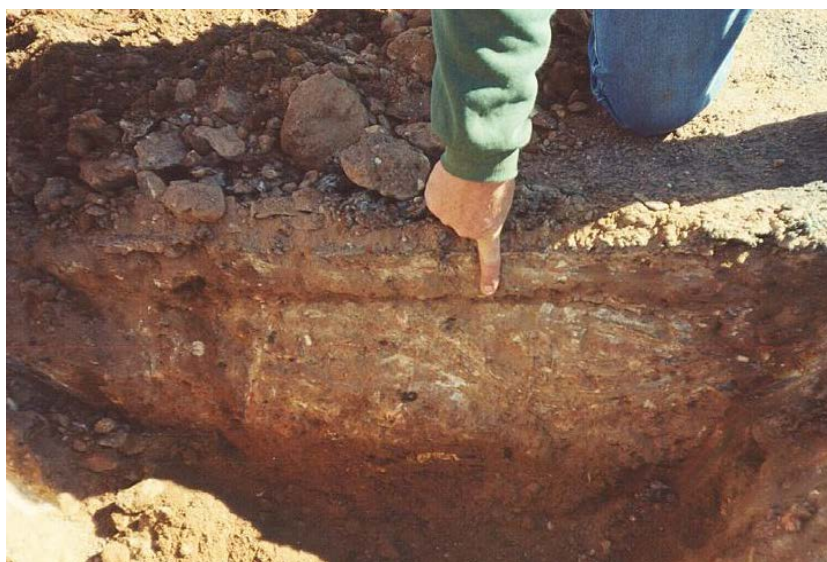
Figure 7.17: Delamination of stabilised material
