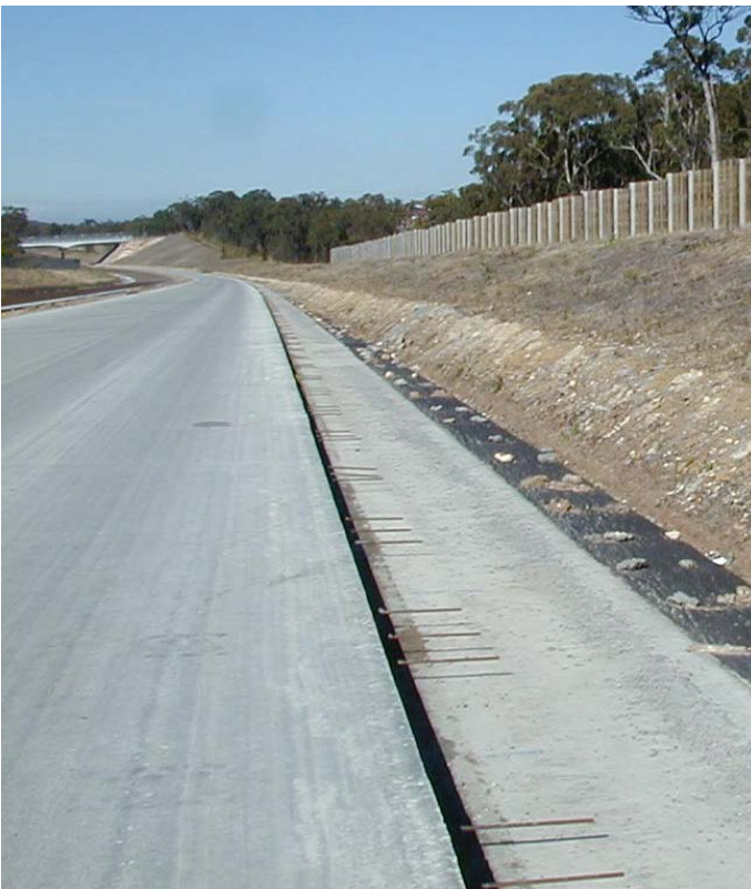
Figure 10.19: Tie bars protruding from concrete slab at longitudinal joint
