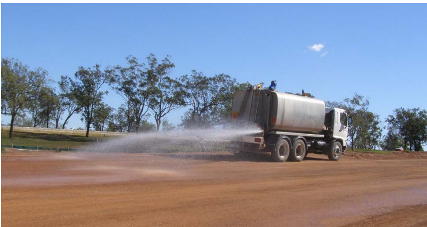
Figure 6.5: Water cart ensuring surface of granular material does not dry out prior to surfacing
