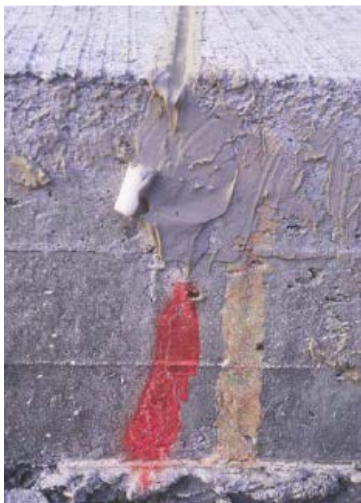
Figure 10.23: Sealant extending down the side of the base concrete
