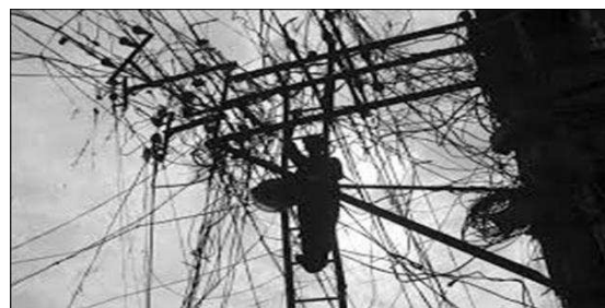
Figure 2: An example of distribution losses due to electricity theft in Pakistan
