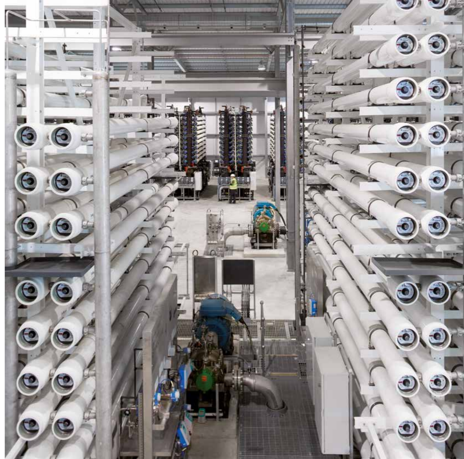
Beckton Desalination Plant, London, United Kingdom
