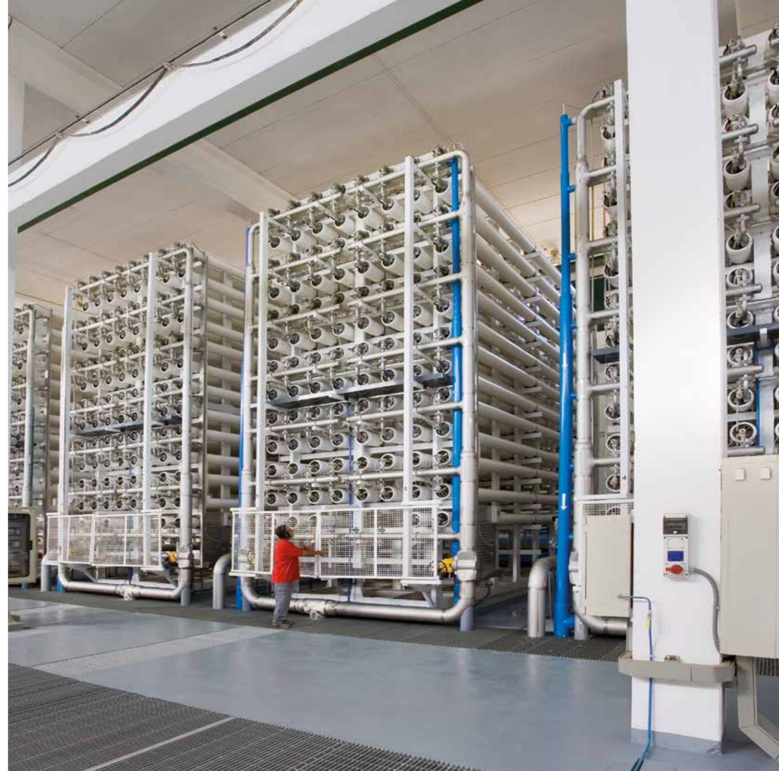
Jávea Desalination Plant, Alicante, Spain
