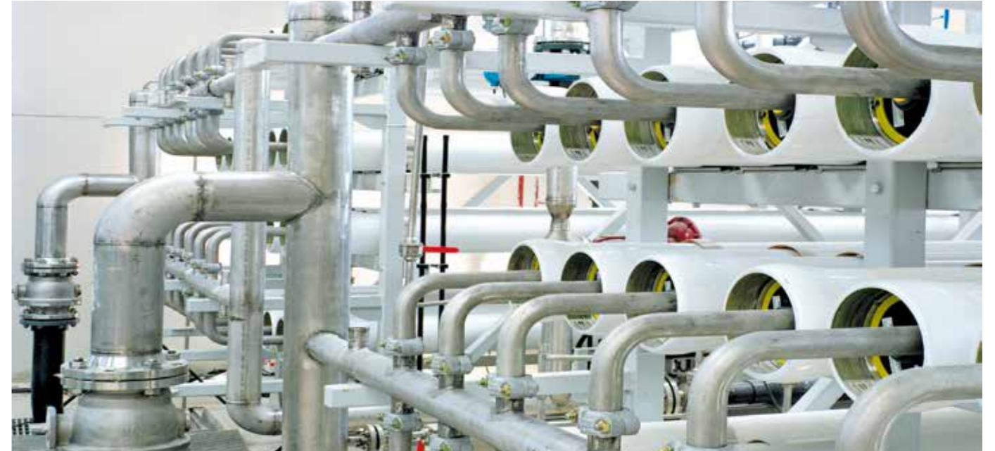
Tertiary treatment of waters from the WWTP in Campo Dalías, Almería, Spain
