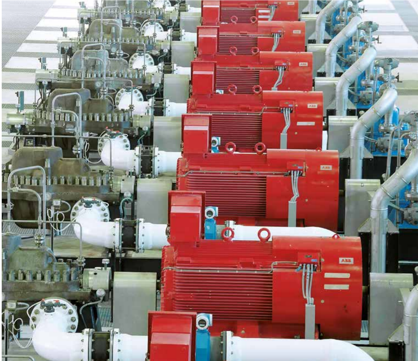
Desalination plant in Alicante, Spain
