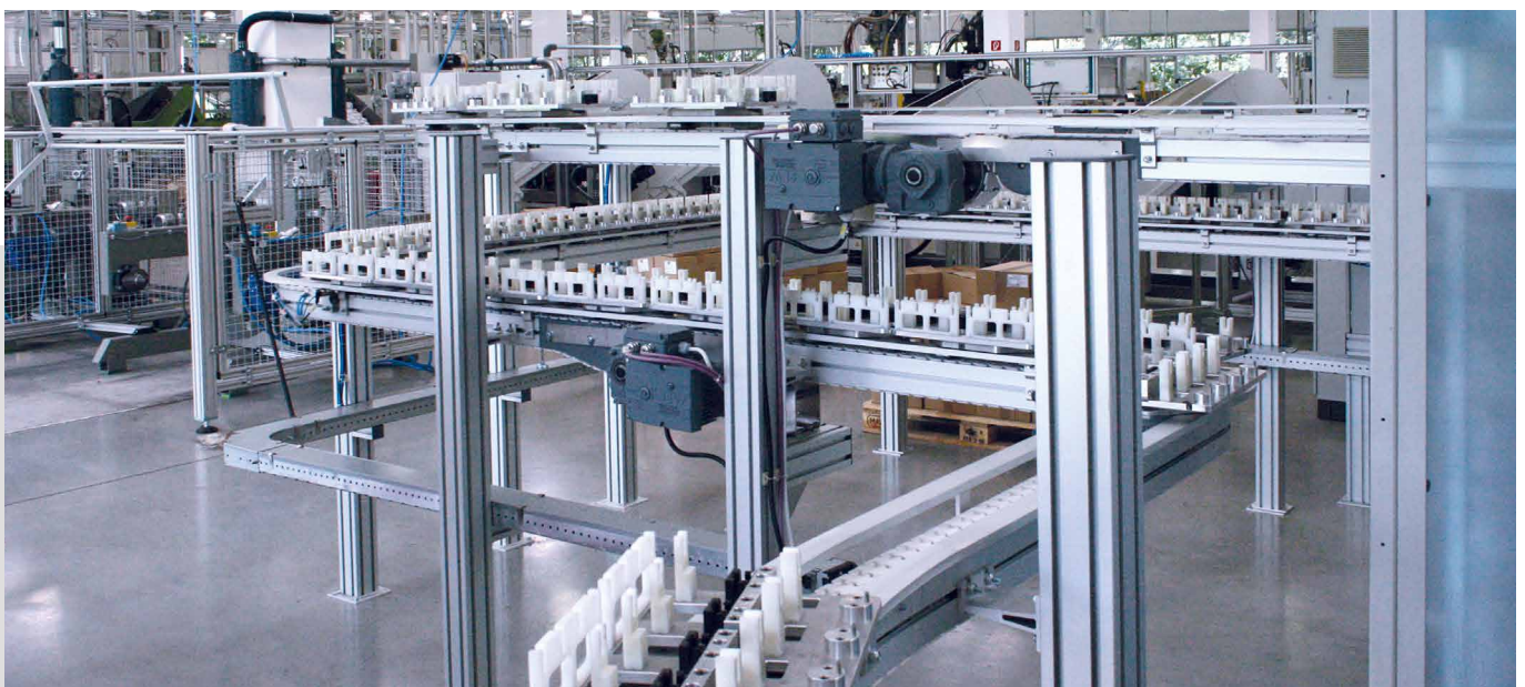
Complex flat top chain conveyor on multiple levels for the transport of pallets
