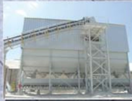
Weigh Belt Plant
