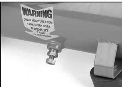
Figure 10. Tank drain valve.
