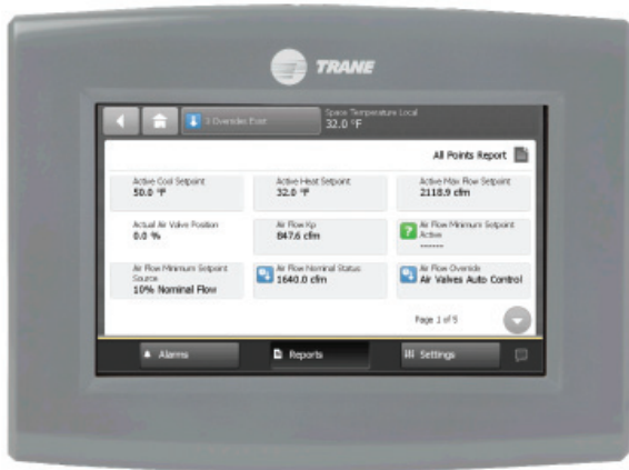
Figure 18 – TD7 operator interface
