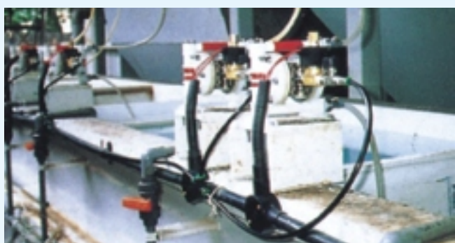
Blagdon 06 moulded pumps being used by Duraco Industries, Singapore, for chemical injection at a waste treatment plant.
