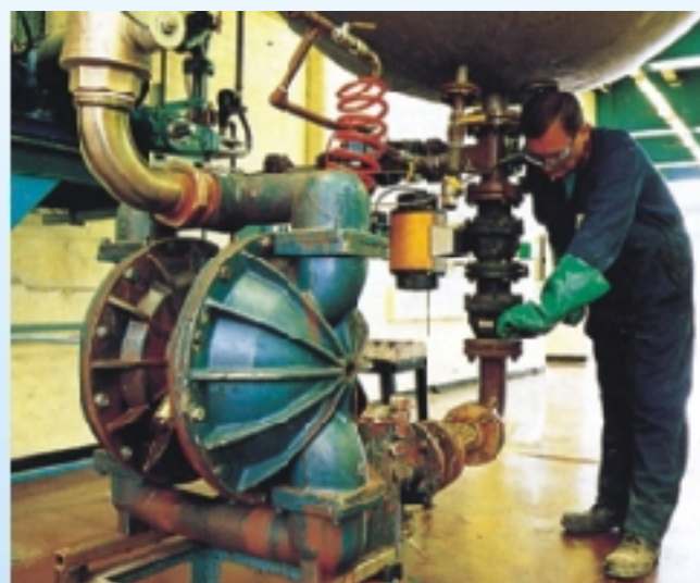
Blagdon 75 pump transferring paint from dispenser to blending vessel.
