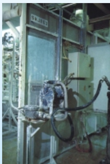
This Blagdon 25 metallic pump at Caradon Bathroom is feeding a robotic spray glazing operation.
