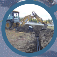
Cables for temporary power distribution
