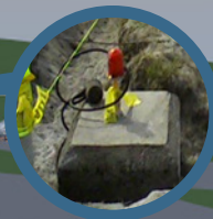
Cables for field transformer
