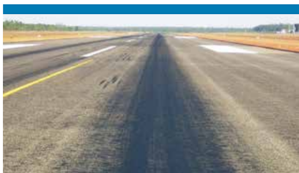
Figure 49: Flushed sprayed seal surface
