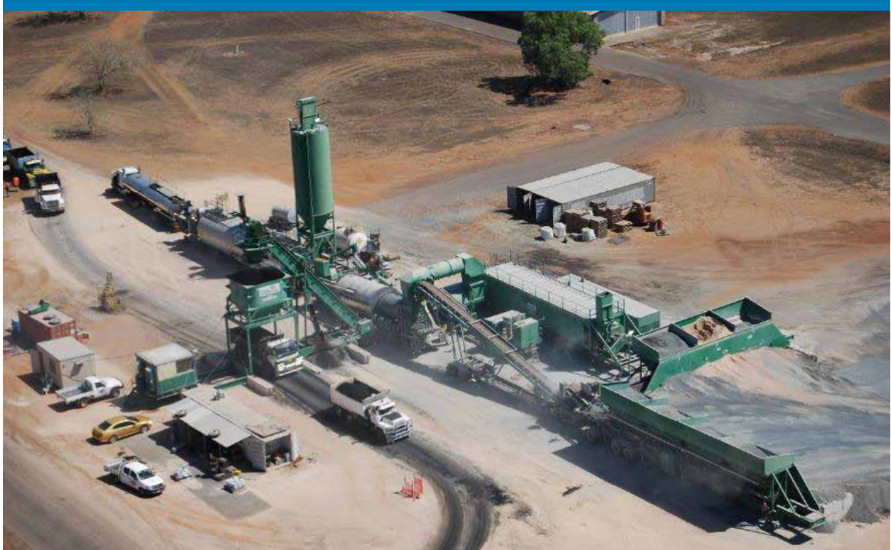
Figure 32: Mobile asphalt production plant
