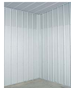
Finished view showing the ceiling enclosed with our optional Hi-Rib acoustical steel
