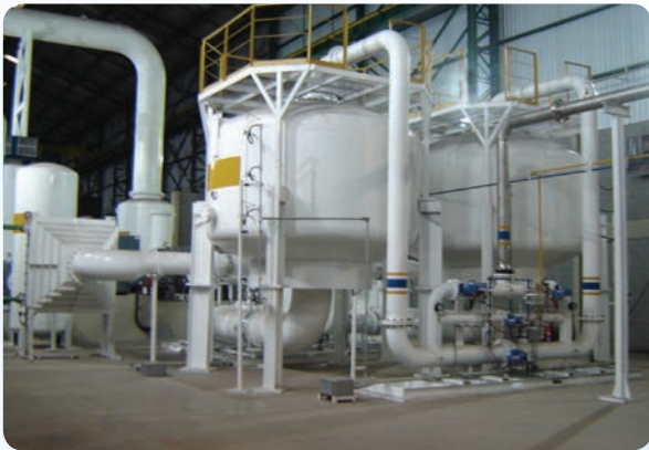
Two ASV80000 VPSA Oxygen Plants at a Steel Mill — Maraba, Brazil
