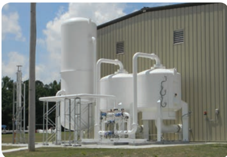
ASV27000 VPSA Oxygen Plant at a Wastewater Treatment Facility — Rocky Mount, NC USA
