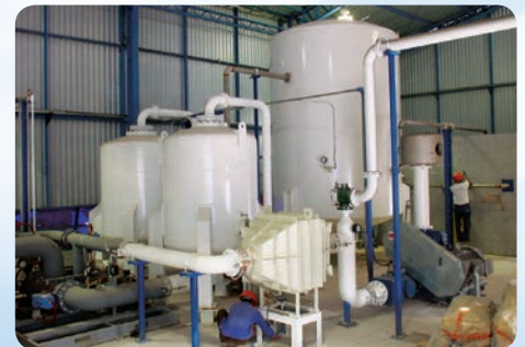
ASV14500 VPSA Oxygen Plant at a Steel Mill — El Salvador
