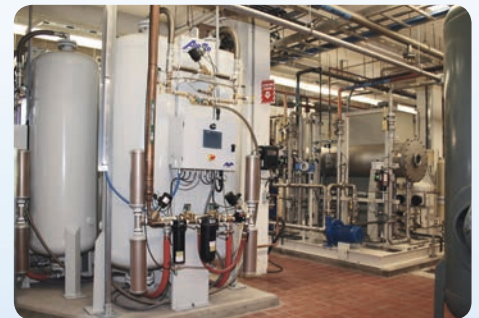
AS-L1000 Triplex PSA Oxygen Plant for ozone generation — St. Jean, Quebec, Canada
