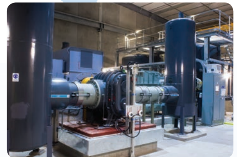
Two ASV39000 VPSA Oxygen Plants for ozone generation — Melbourne, Australia
