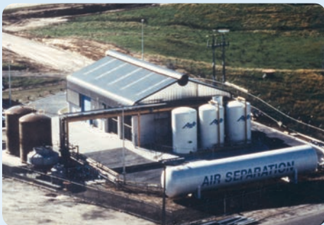
Installed and in operation at a Pulp and Paper Mill since 1991, this 42 TPD PSA Oxygen Plant supplies gas for bleaching and delignification.
