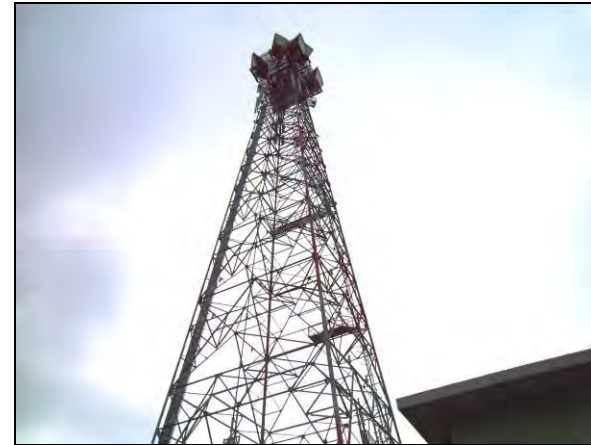
Microwave Transmission Tower
